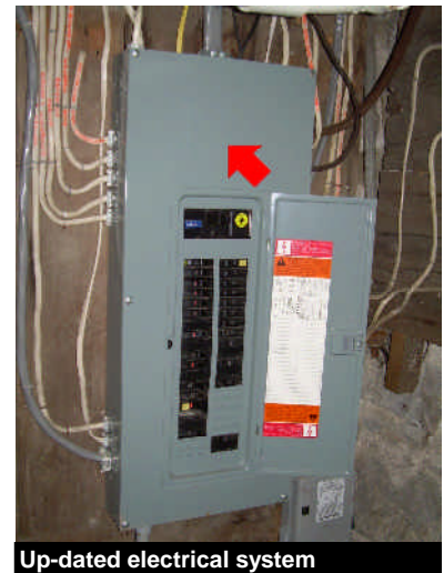
Up-dated electrical system
